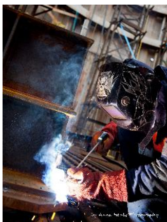
A welder works at the base of the South Tower before a concrete pour.
